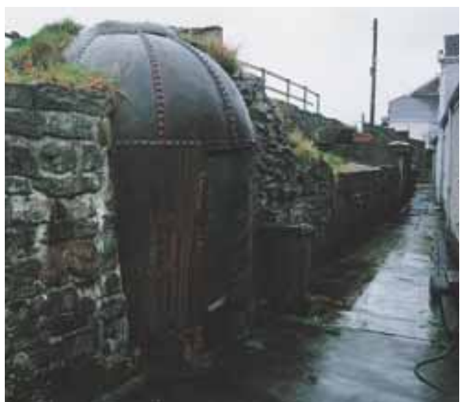
Opposite and left: Work to halt erosion of the river bank at Skenfrith, Monmouthshire. Above: A haystack boiler in use as a shed at Abercanaid, Merthyr Tydfil.
