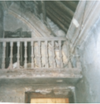
Above: Eagle Academy, Cowbridge. The gallery before restoration. Below: Interior and exterior completed.
